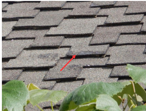
Deterioration at surface
