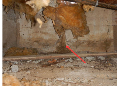
Moisture stains at foundation
