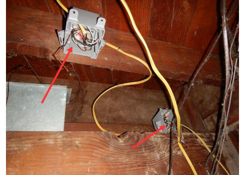
Open junction boxes
