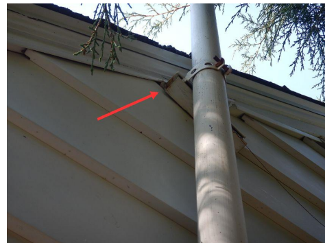
Conduit appears loose
