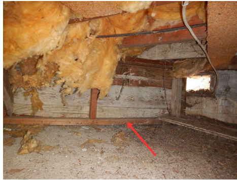
Earth to wood contact in crawl
