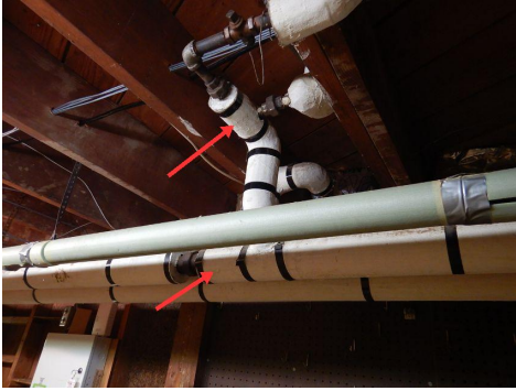
Older covering may contain asbestos
