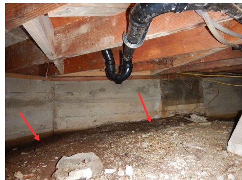
Moisture in crawlspace
