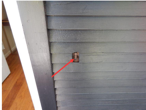
Improper exterior switch
