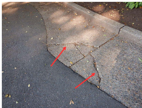
Trip hazards at driveway
