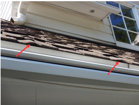
Lifting and loose shingles
