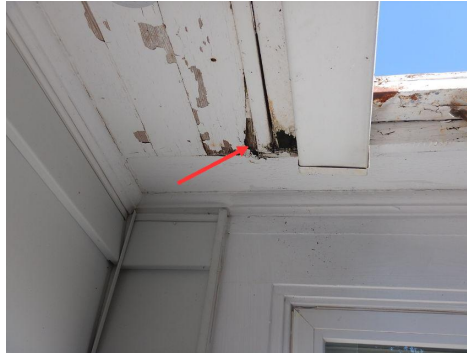
Possible leak at metal roof
