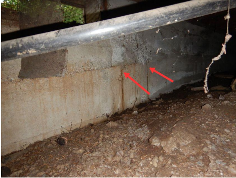
Moisture stains in crawlspace
