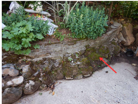
Displacement at wall
