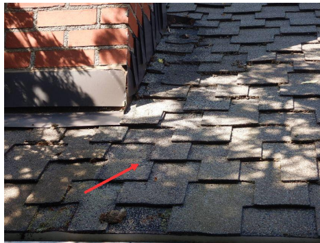
Deterioration at surface
