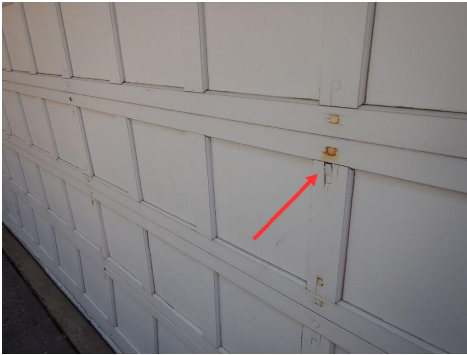
Heavy wear at door
