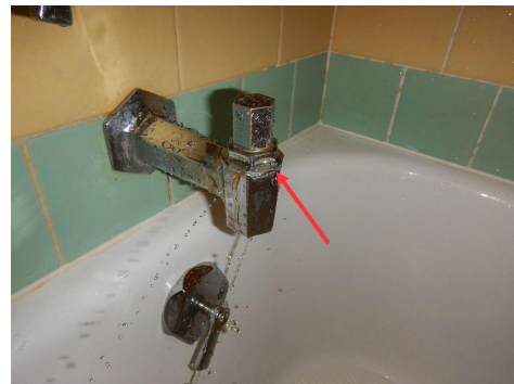
Diverter not operating properly
