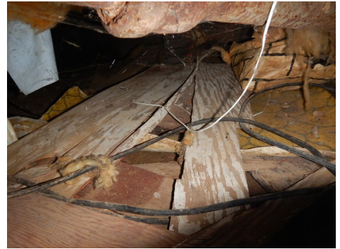
Debris in crawlspace
