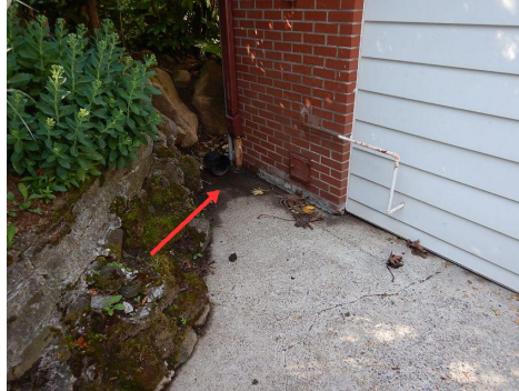
Poor drainage at patio
