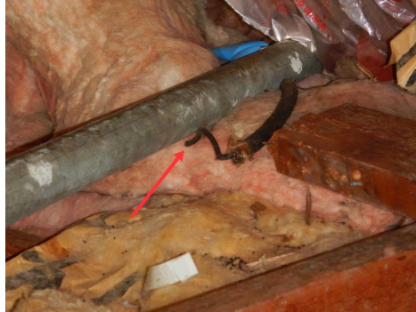
Abandoned wiring in attic
