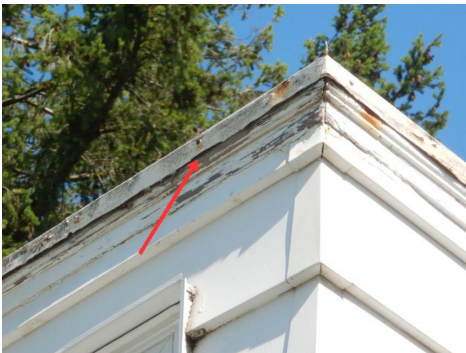
Wear at fascia
