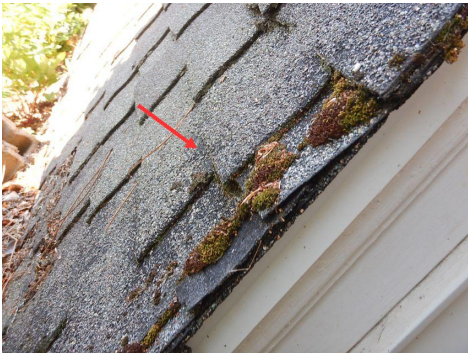
Heavy wear at roof
