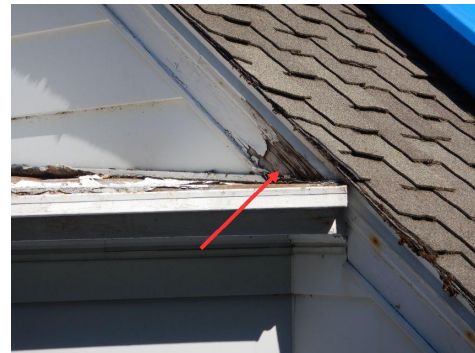
Moisture damage at roof edge
