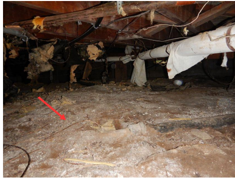
Exposed soil in crawlspace
