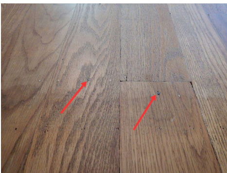
Nails lifting at floor
