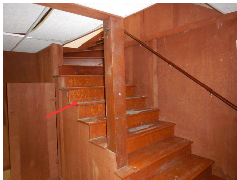
No railing at side
