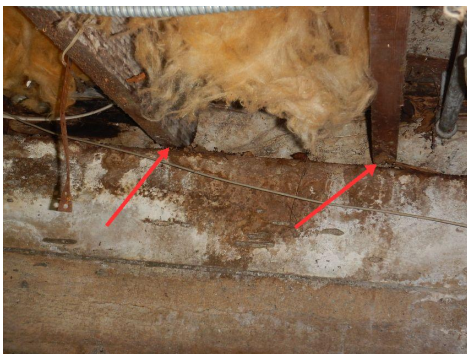
Significant rot and insect damage
