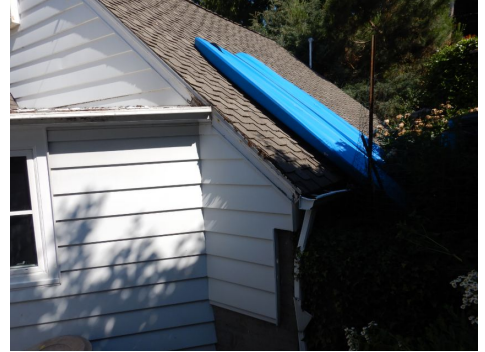
Stored items on roof
