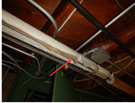
Damaged covering may contain asbestos
