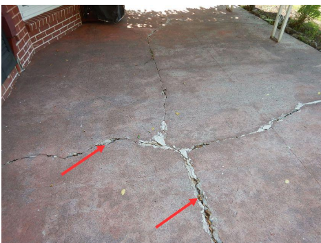
Large cracks and trip hazards
