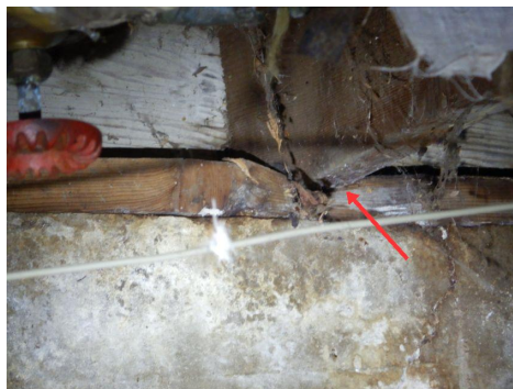
Significant rot and insect damage
