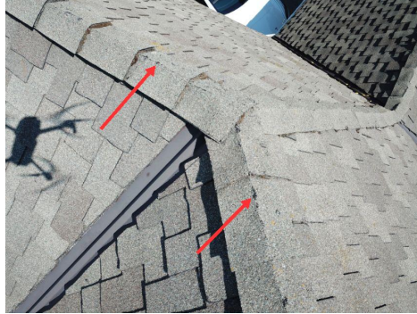
Damaged ridge shingles
