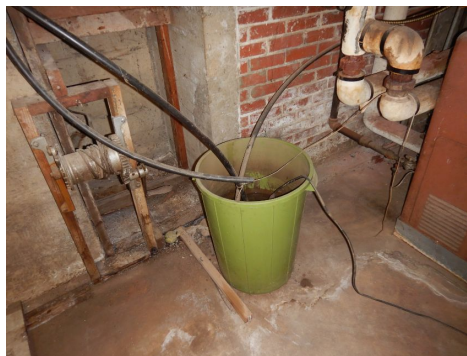
Pump system in basement
