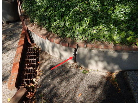
Large crack at wall
