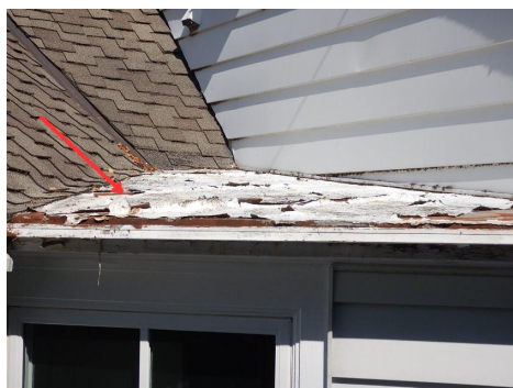
Heavy wear at metal roof
