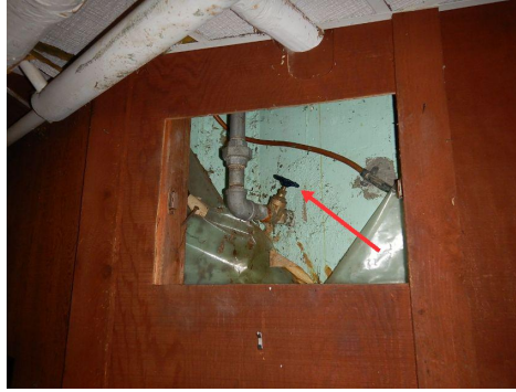
Shut off in basement
