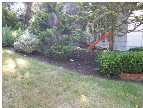
Improper drainage in areas
