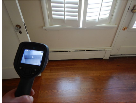
Radiator not heating
