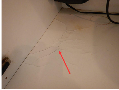
Moisture damage under sink
