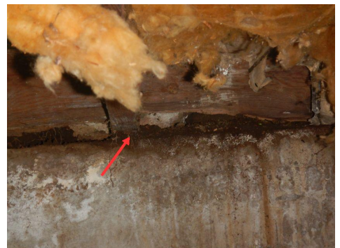
Significant rot and insect damage
