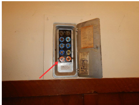
Fuses at obsolete panel
