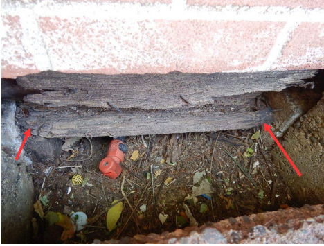
Rot at vents
