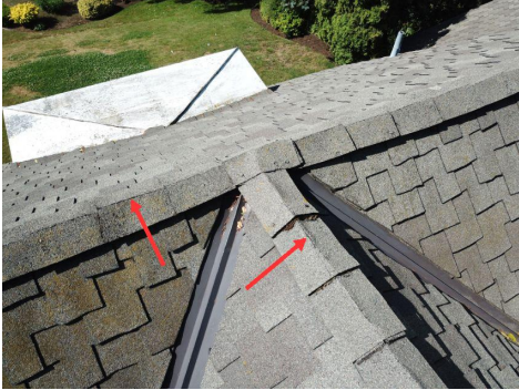
Damage at ridge shingles
