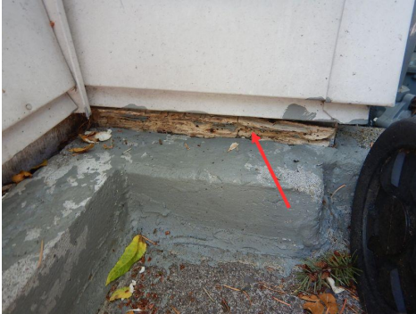
Rot at wall
