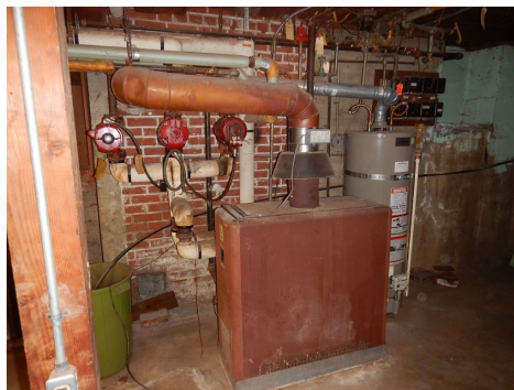
Boiler needs evaluation
