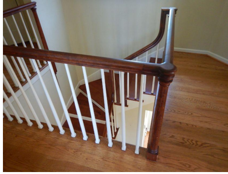
Low fall railing, openings too wide
