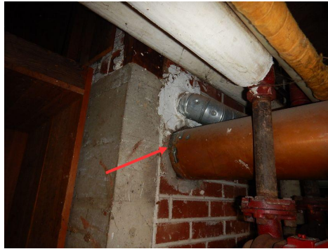
Boiler venting into unlined chimney
