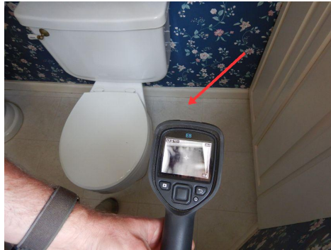
Evidence of moisture in floor
