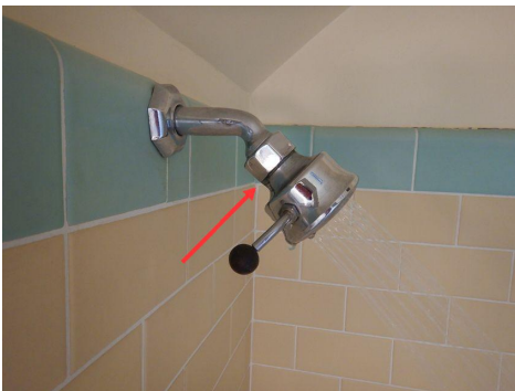
Shower head leaking
