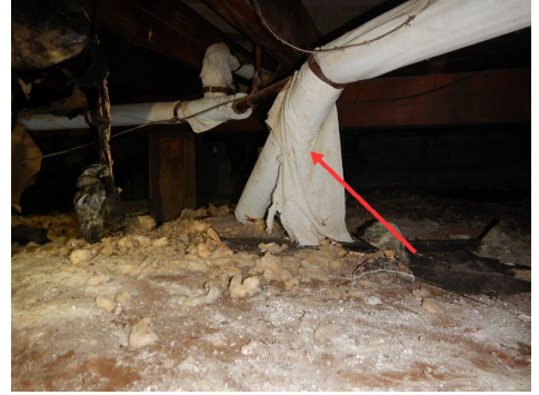
Damaged covering may contain asbestos
