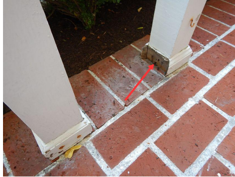
Rot at post
